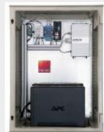
Power Plant Controller
